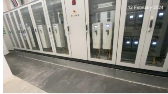
Electricity panel with rubber mat.JPG
